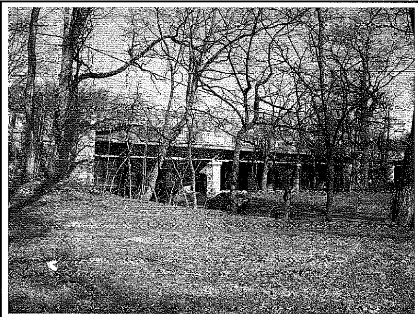
Route 4 Bridge over Palisade Avenue/CSX Railroad/Windsor Road. This photograph shows the western spans viewed from South Gaylord Park. Windsor Road is visible at center, and Windsor Park is located on the opposite side of the road.
